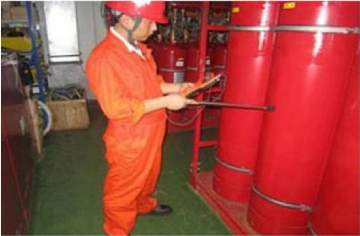
For CO2 storage tank of the fire fighting system in the offshore drilling platform.
